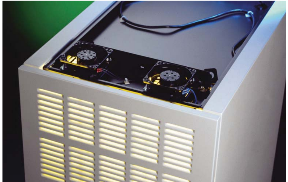
Extractor fan installed in rack
